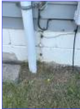
The panel is grounded to a driven rod.
