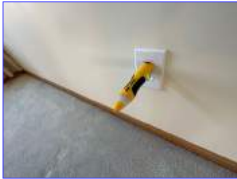
The outlets that were tested are functional.
