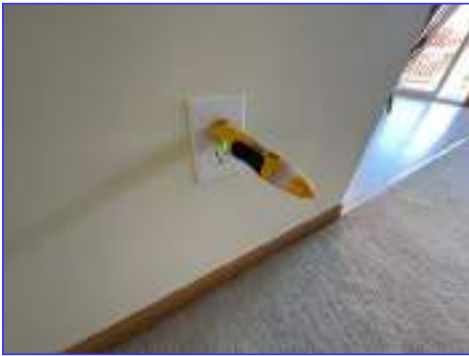
The outlets that were tested are functional.
