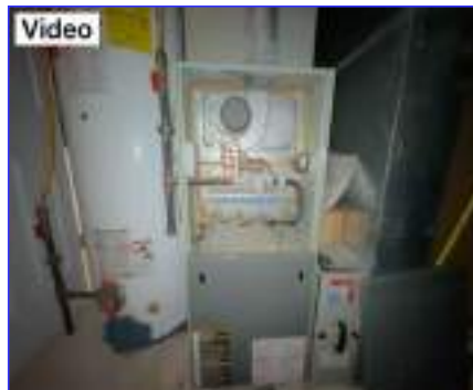
Combustion chamber OK
