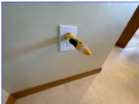
The outlets that were tested are functional.
