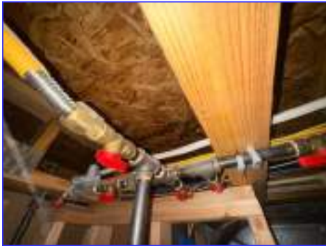
The csst (corrugated stainless steel tubing) in the home were not bonded
