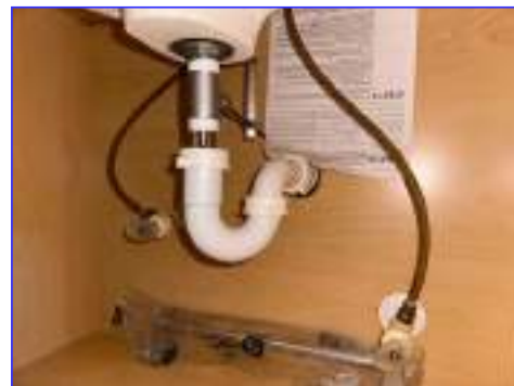
The drain assembly appears to be in satisfactory condition with no visible leaks or deficiencies.
