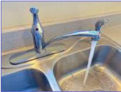
The Faucet is functional.
