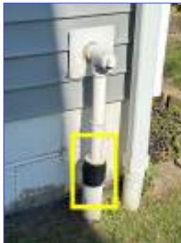
The sump pump discharge pipe is damaged, improperly repaired with duct tape and should be serviced or replaced.
