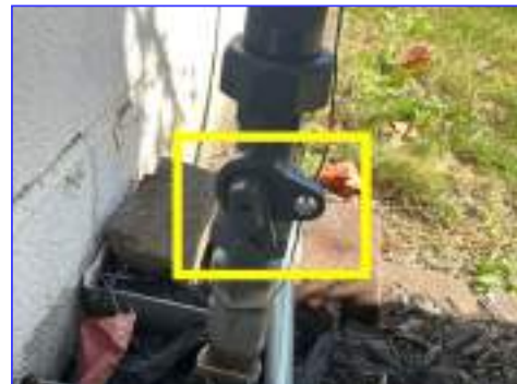
Main gas shut-off.
