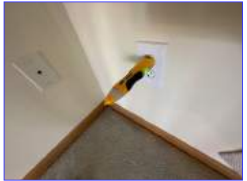
The outlets that were tested are functional.
