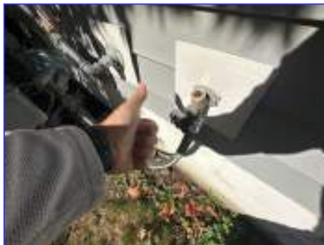
The exterior faucets are functional.
