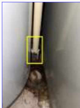
The pressure relief valve was leaking
