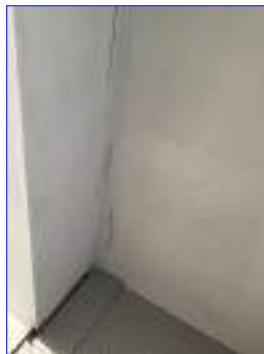
Cracking and peeling observed, recommend review for repair. No water stains observed at the time of inspection.
