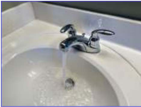
The Faucet is functional.
