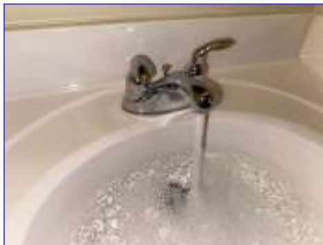
The Faucet is functional.
