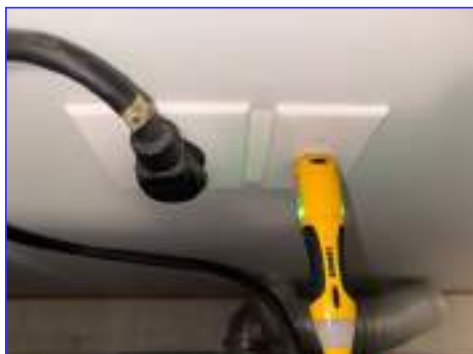
No ground fault circuit interrupter (GFCI) protection of electrical receptacles observed.
