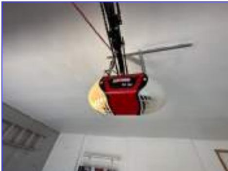
The garage door opener is functional.
