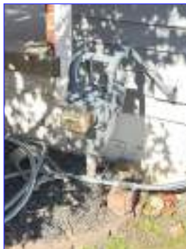
The gas main shut-off is located at the meter in the side yard.
