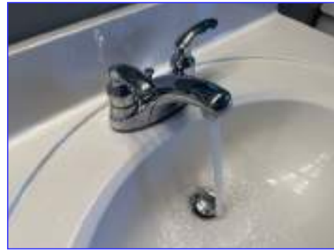
The Faucet is functional.
