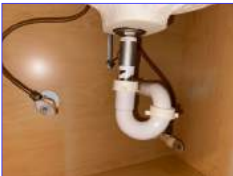
The drain assembly appears to be in satisfactory condition with no visible leaks or deficiencies.
