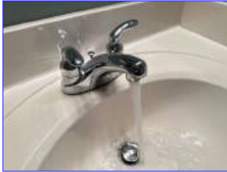
The Faucet is functional.
