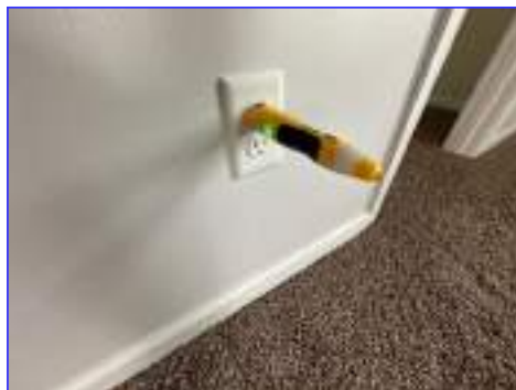
The outlets that were tested are functional.
