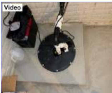
The sump pump is accessible and in acceptable condition.
