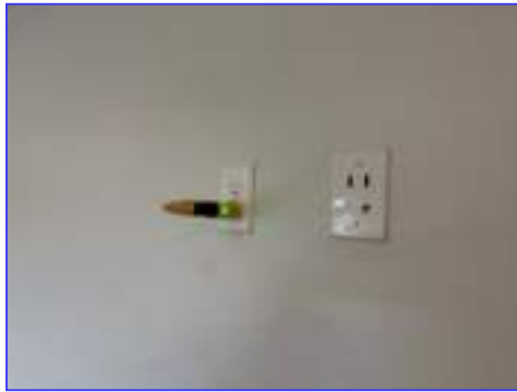
The outlets that were tested are functional.
