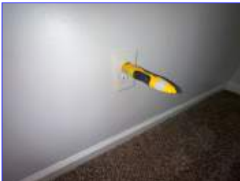
The outlets that were tested are functional.
