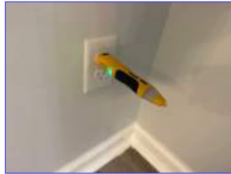
The outlets that were tested are functional.
