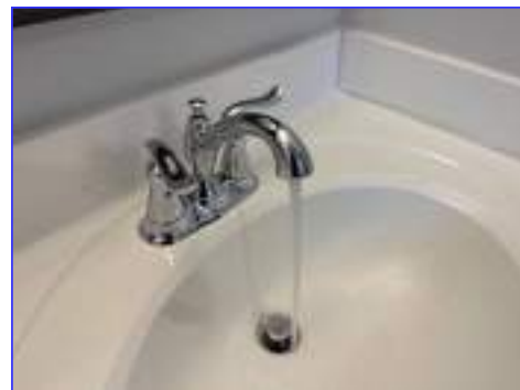
The Faucet is functional.
