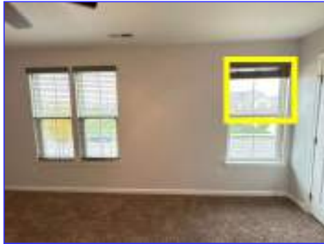
Broken hermetic seal.
