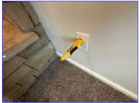
The outlets that were tested are functional.
