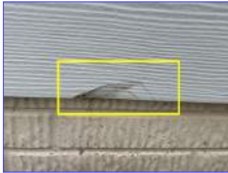
Isolated cracks and damage observed.
