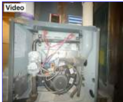
Combustion chamber OK
