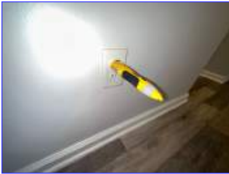
The outlets that were tested are functional.
