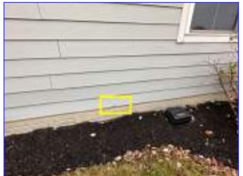
Isolated cracks and damage observed.
