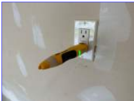
The outlets are functional and include ground-fault protection
