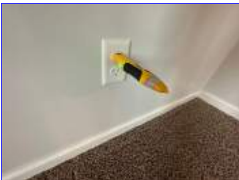
The outlets that were tested are functional.
