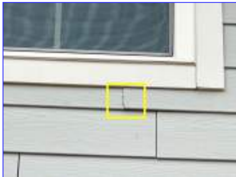
Isolated cracks and damage observed.
