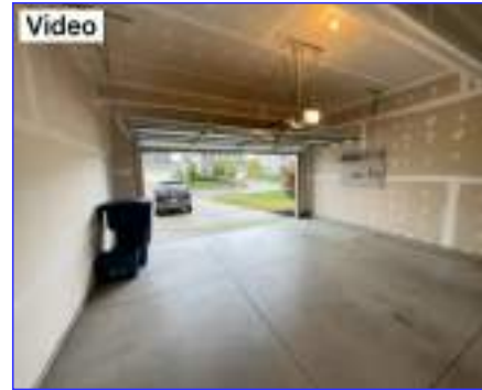
The garage door opener is functional.
