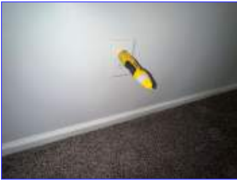
The outlets that were tested are functional.
