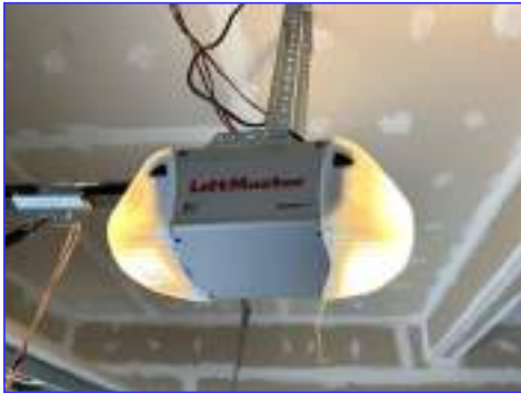
The garage door opener is functional.
