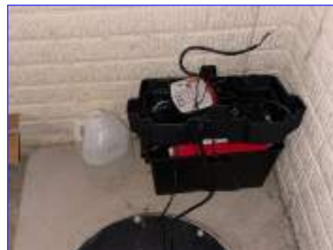
||4||The back up pump does not appear to be in service.
