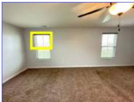
Broken hermetic seal.
