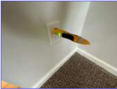
The outlets that were tested are functional.
