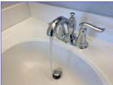
The Faucet is functional.
