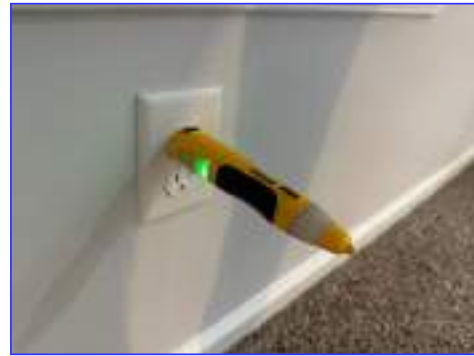
The outlets that were tested are functional.
