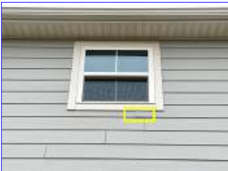
Isolated cracks and damage observed.
