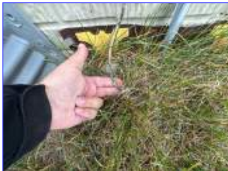
The panel is grounded to a driven rod.
