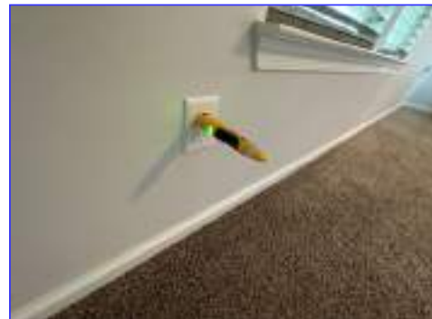
The outlets that were tested are functional.
