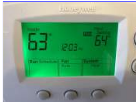
Thermostat settings upon completion
