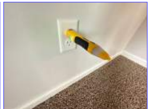
The outlets that were tested are functional.
